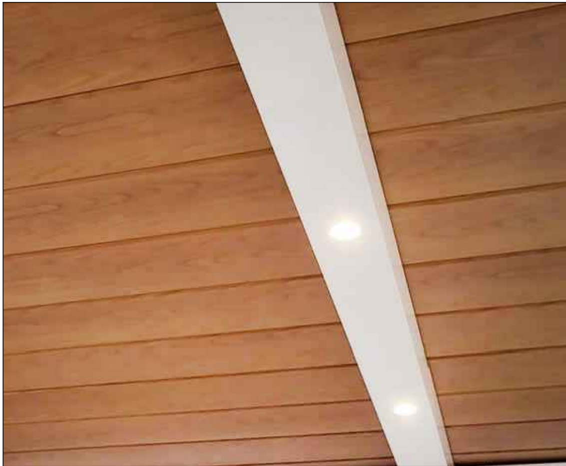
PERGOLA RECESSED DOWN LIGHTS
